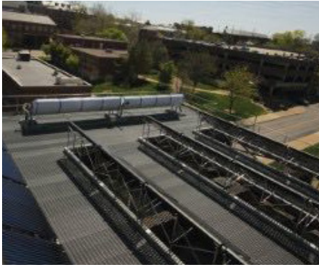
Installed Solar Panels at the University of Missouri
