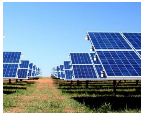
Installed Solar Panels at the University of Tennessee
